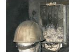
BOP ENERGY 3000 after arc flash incident
